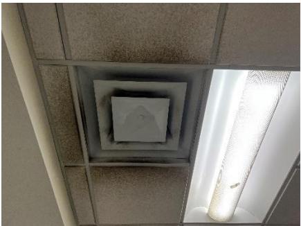
7. Room 3.02.04, Dirt and limited mold
