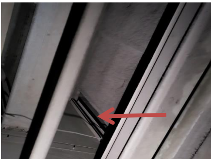
10. AH 1, Improperly seated filters
