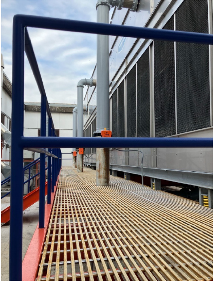
Buena Vista District Cooling Tower
