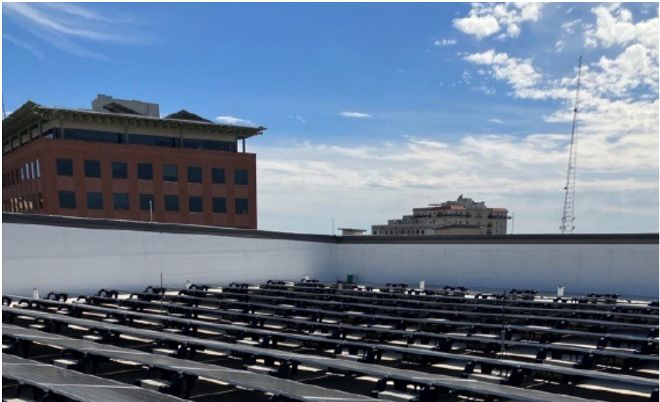
San Pedro I Rooftop Solar
