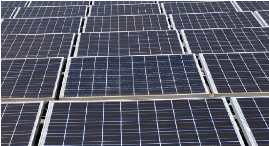
San Pedro I Rooftop Solar
