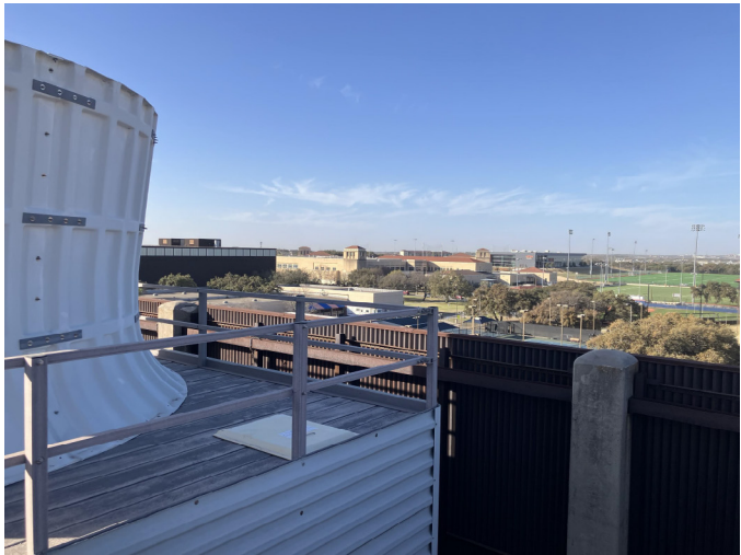
North Thermal Energy Plant Cooling Tower
