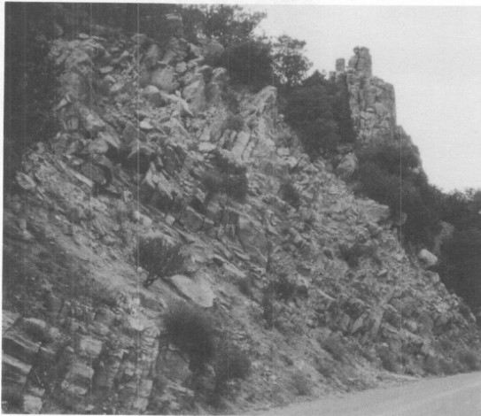
Figure 5. This picture demonstrates a slope profile that has minor launching features that could cause rockfall. This would have a RHRS rating of 9 points.
