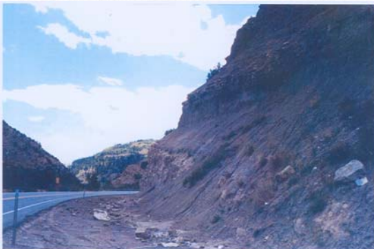
Figure 6. This picture is showing many launching features that could result in rockfall. This would have a RHRS rating of 27 points
